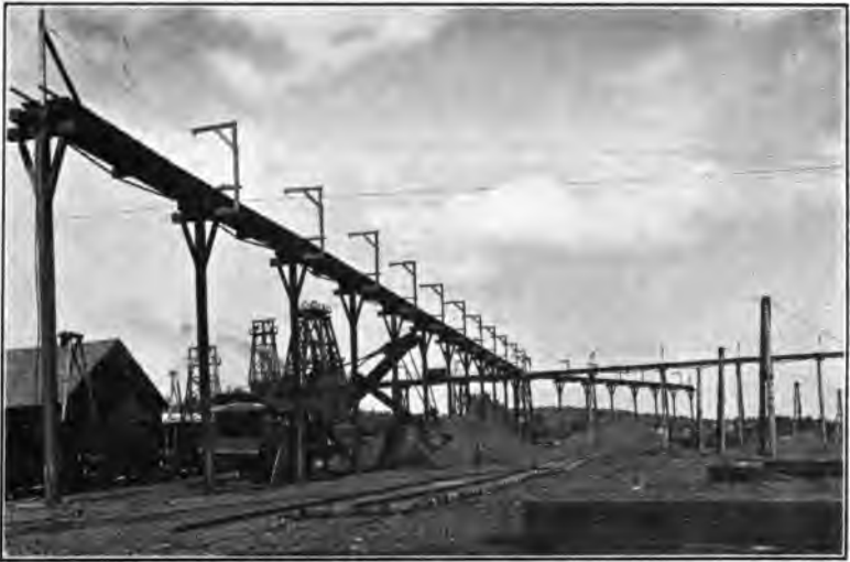
STEAM SHOVEL WORKING ON LAST OR CLEAN-UP CUT. SHOVEL WORKING BETWEEN BENTS.
